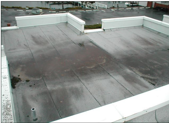
Standing Water North Side
