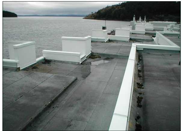
Standing Water South Side
