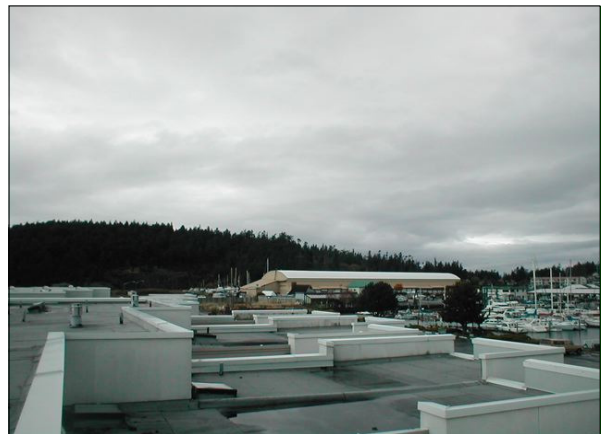
Standing Water Along North Roof
