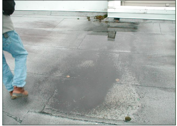
Typical Standing Water and Eroding Roofing Particles
