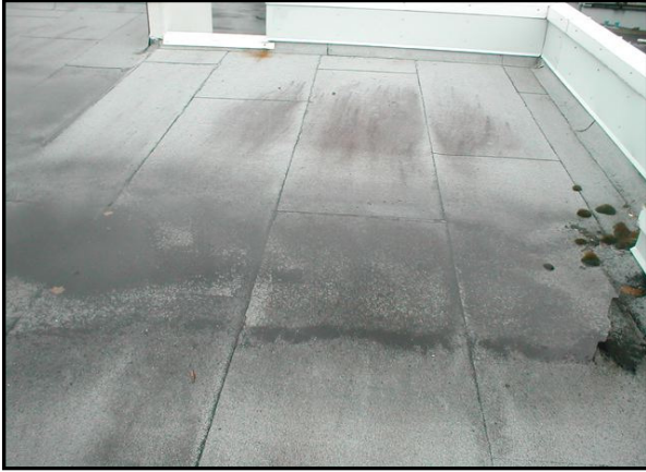
Typical Standing Water
